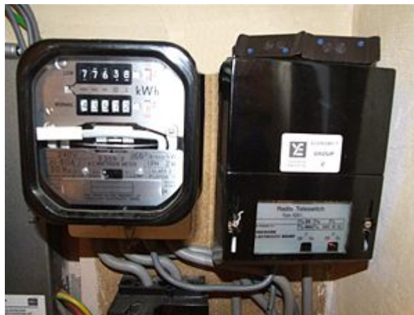
Economy 7 Meter and Teleswitcher
